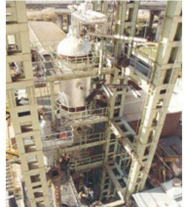
GEST plant vessel (volume 43 m 3 , height 15 m)
