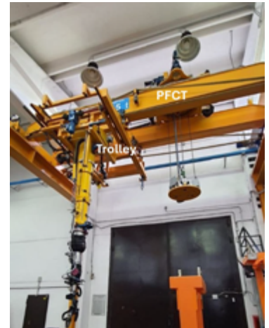
DRP hall – Carroponte, trolley e PFCT
