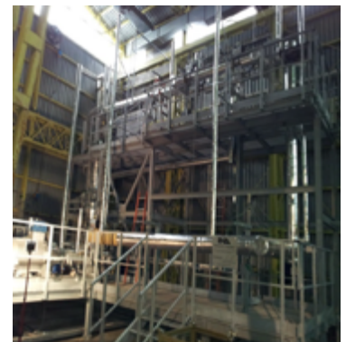
HELENA facility: the FIVFPS test section at the top, and the primary circuit at the bottom
