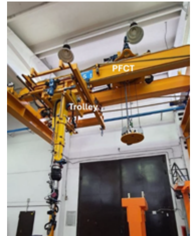
DRP hall – Gantry Crane, trolley and PFCT
