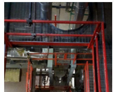
SIRIO facility: tests on a passive DHR system for the ALFRED LFR
