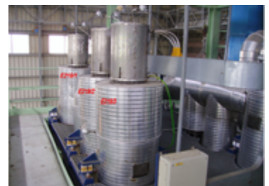
HeFUS3 facility: the turbo-circulator section, at the top, and the electrical heaters, at the bottom.
