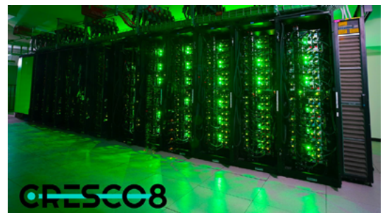
The CRESCO 8 Supercomputer.
