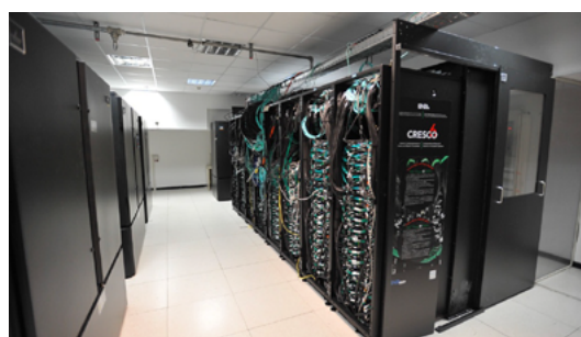
The CRESCO 6 Supercomputer.
